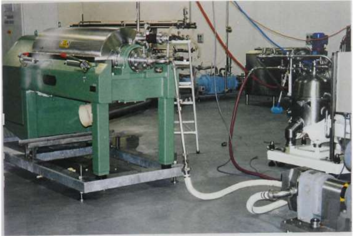
Appendix IV Decanter (left) and clarifier (right) centrifuge.
