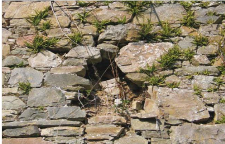
Figure 2.13: Deteriorated mortar that has ultimately led to the loosening and collapse of rubble masonry.
