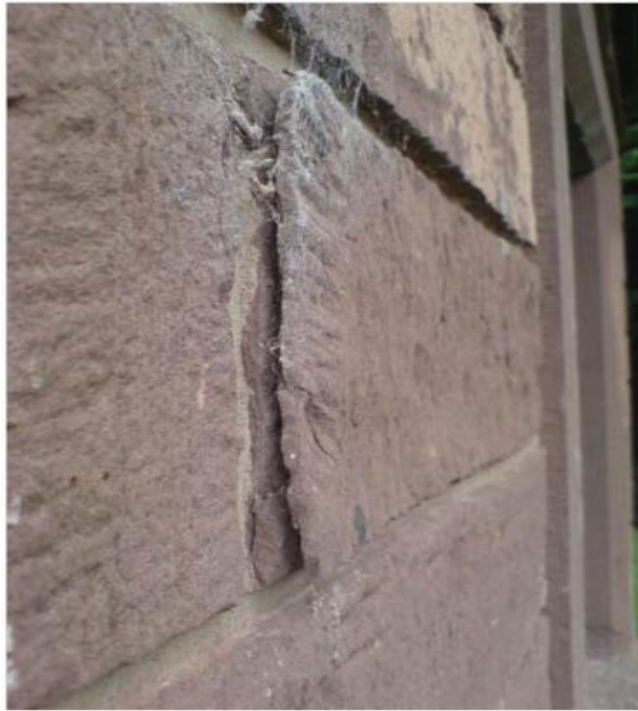
Figure 2.17: Delaminating argillaceous (clay rich) sandstone, Doune Castle Source: Forster, 2010b.
