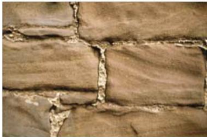
Figure 2.12: Loose joint of rubble stonework
