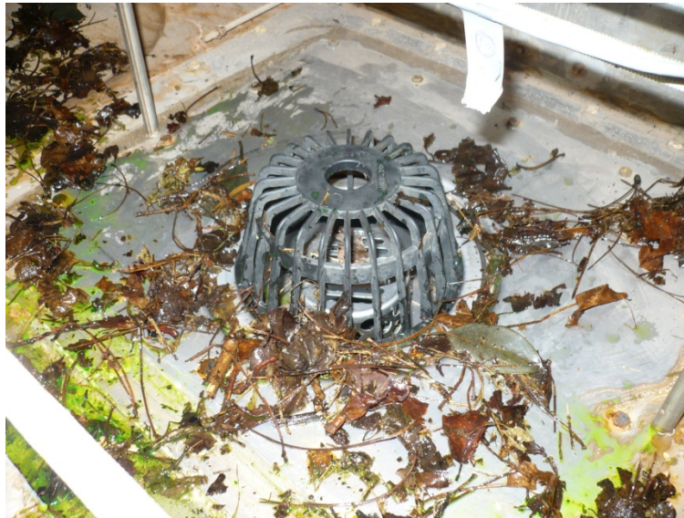
Figure 5.4(a) Outlet B, before loose detritus test.
