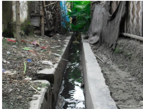
Railway Slum: In Railway slum, drainage facility was provided by LPUPAP. Due to the lack of disposal point, this drainage does not work in the heavy rain and causes water logging in the area.
