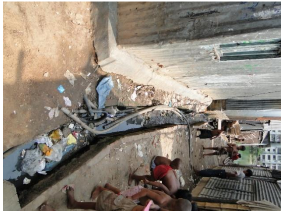
Karail Slum: In Karail, the drainage facilities were developed under the SIP and due to the lack of maintenance and management the drainage system remains blocked and water disposes in the neighbouring lake.
