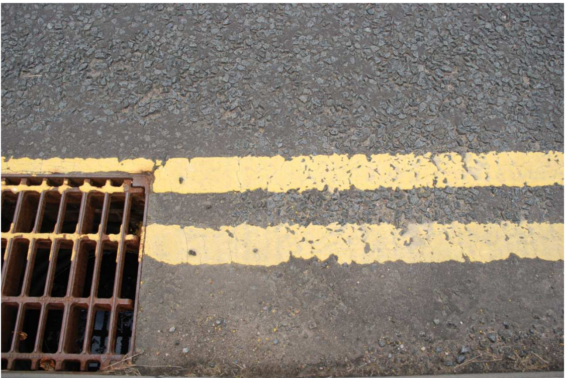
Site 2: Straight road section on link road between Boundary Road North and Research Avenue North Road
