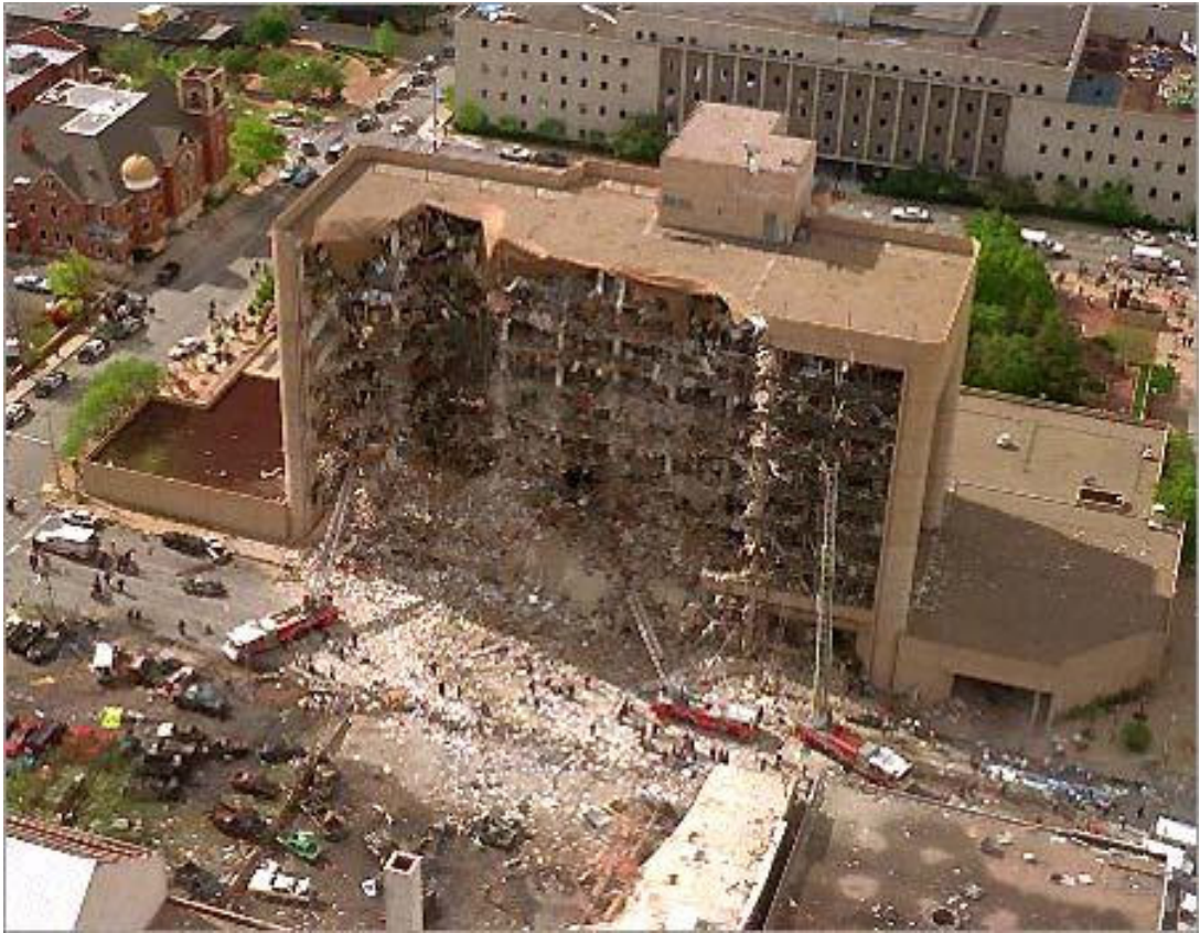
Figure 3.3a: Damage to the Alfred P. Murrah Federal Building in Oklahoma City 1995, after AP the Associated Press
