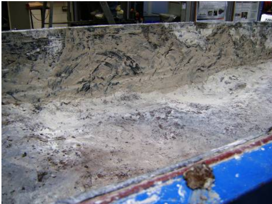
Figure 5.40. Erosion of formation under centre sleeper
