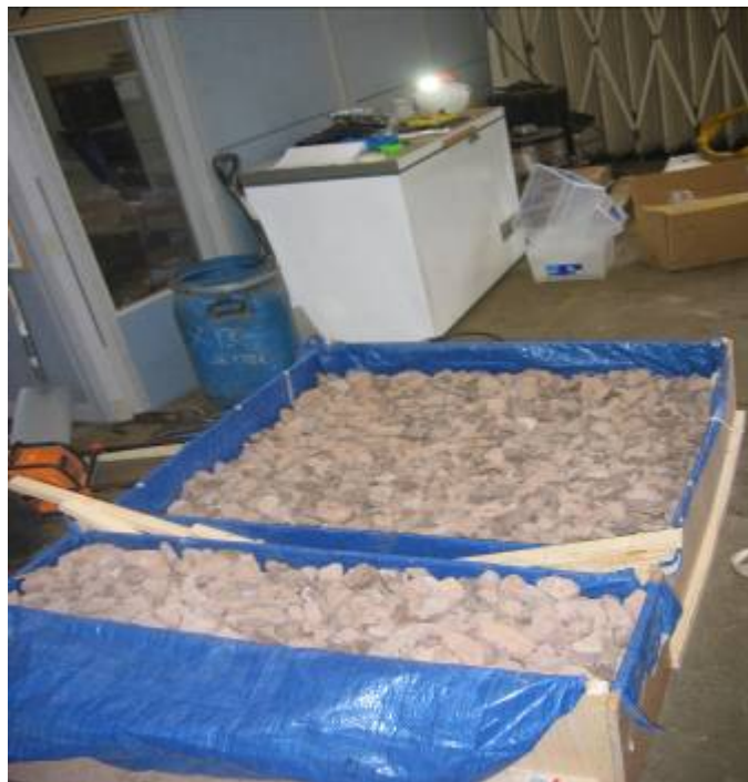
Figure 5.9. Additional ballast slab and beam sections prior to the application of the XiTRACK polymer
