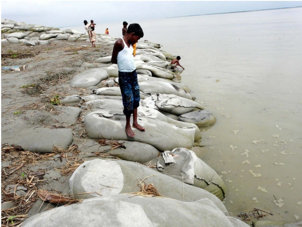
(c 1) Inadequate thickness of geobag revetment
