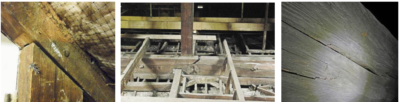
Figure 6. Mechanical damage in Trussed roofs. From left to right: joint disconnection in Fort George Ordnance Store (Ardersier, Highland), joint disconnection in Oakshaw Trinity Church (Paisley, Renfrewshire), crack in rafter in Glasgow Trades Hall.
