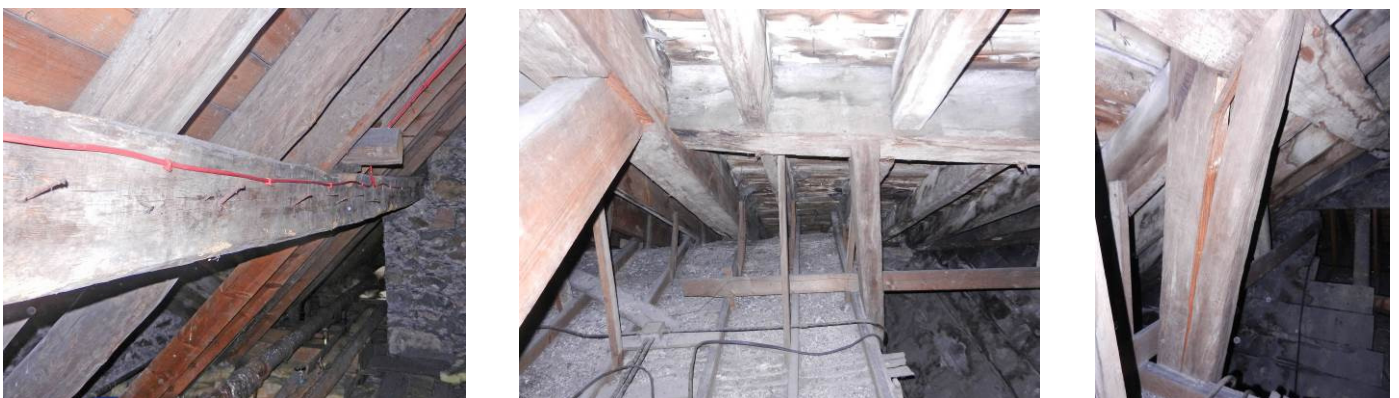
Figure 7. Mechanical damage in purlin roofs. From left to right: deflected purlin in Melville House (Monimail, Fife), deflected purlin in Touch House (St Ninians, Stirling), crack in strut in Touch House (St Ninians, Stirling).
