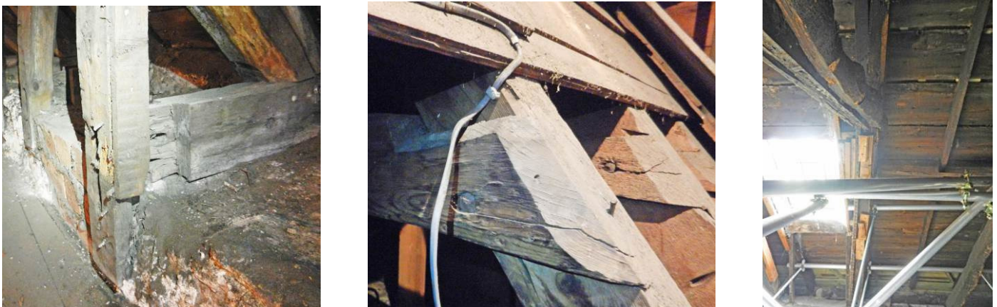
Figure 5. Mechanical damage in common rafter roofs. From left to right: joint disconnection in Sailor's Walk (Kirkcaldy, Fife), joint splitting in Touch House (St Ninians, Stirling), stacking up in Geilston House (Cardross, Argyll and Bute).
