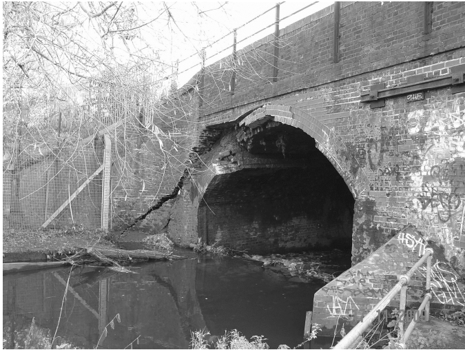
Figure 1. Upstream face of Bridge RDG1 48 showing failed arch following debris blockage (after RAIB 2010).
