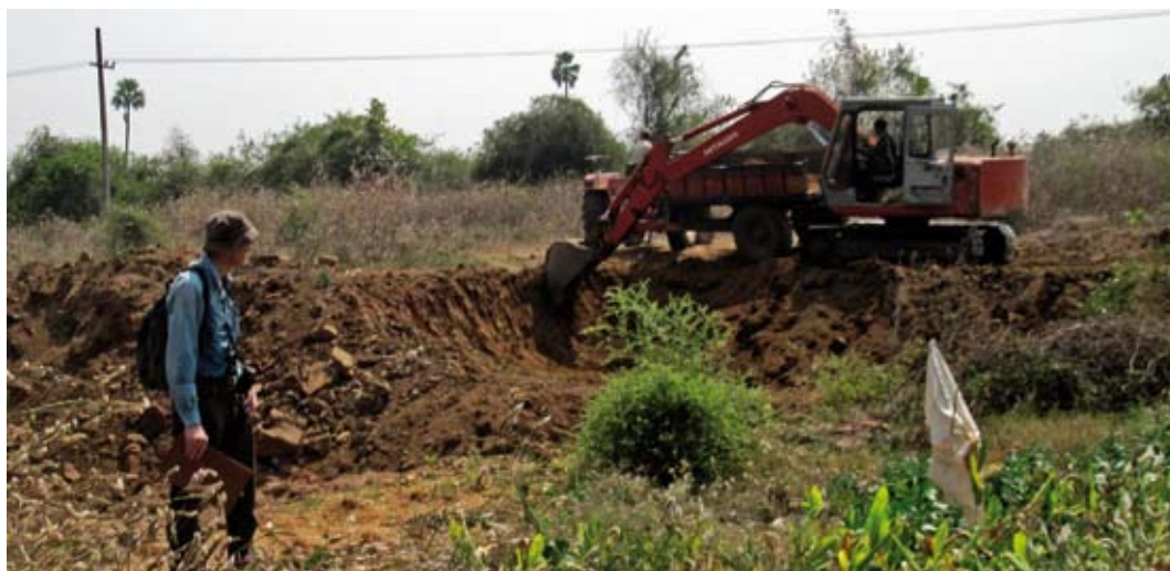
Fig. 5 Many sites were found to be recently damaged or destroyed by land clearance activities. This site was being bulldozed on the day of the survey visit.
