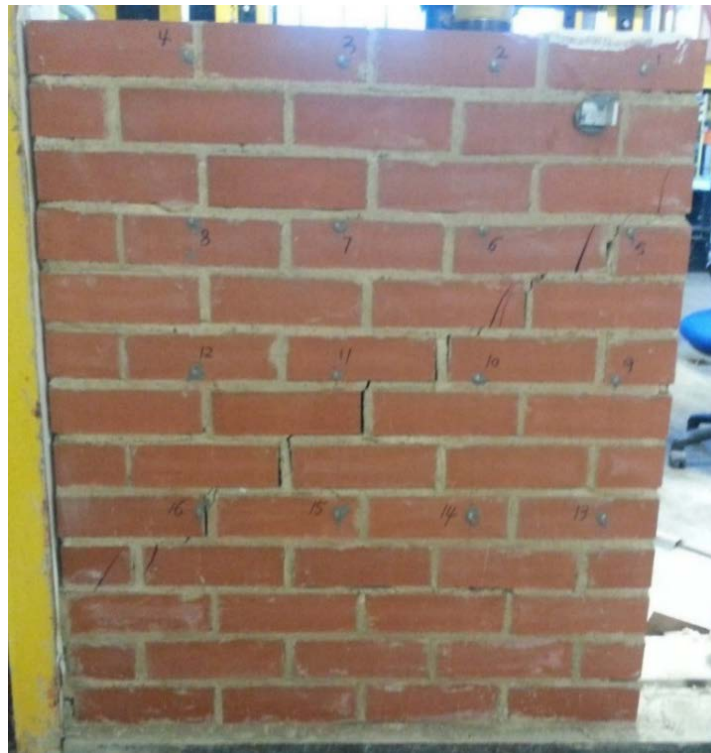
Figure 4.5 Failure pattern of double leaf wall W4 on the loaded leaf
