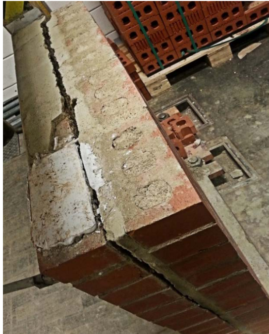
Figure 4.13 Failure pattern of the collar joint on top side of W7
