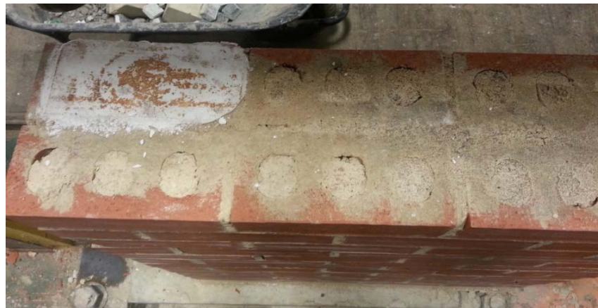
Figure 4.11 Failure pattern of the collar joint on top side of W4
