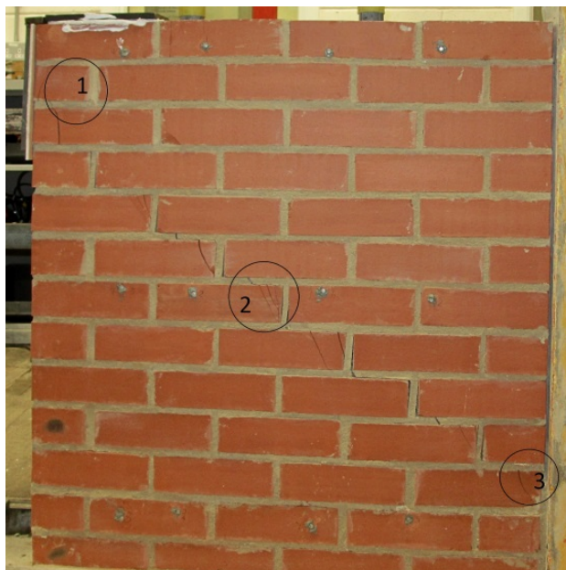
Figure 4.1 Failure pattern of single-leaf Wall 1
