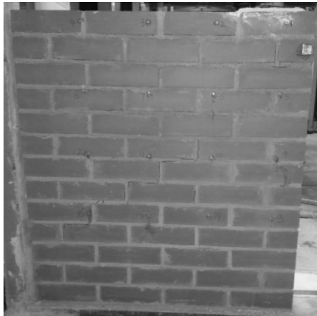
Figure 7.17 Cracks on first leaf in experimental results
