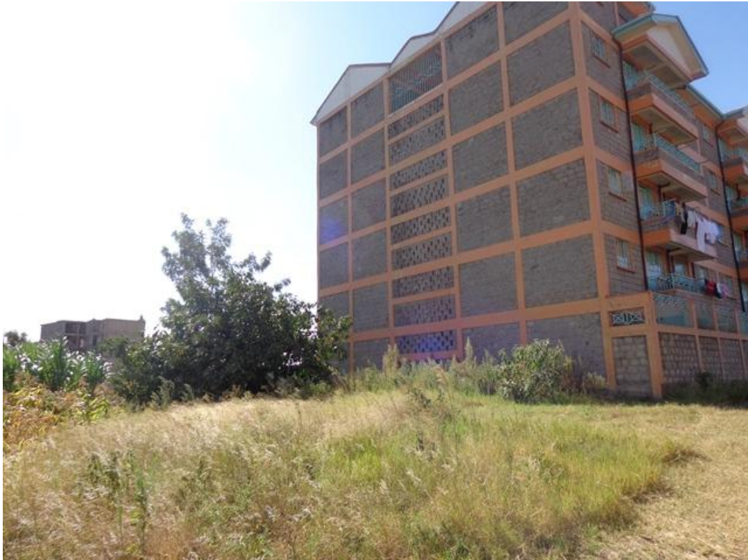
Figure 29: Another apartment block in Kasarani, clearly exceeding the allowable plot ratio (Author, 2014)
