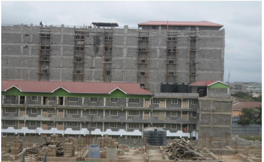
Figure 16: A development under construction in Embakasi area – still going up. The roofed one at the front would be within planning guidelines for the plot ratio (Author, 2014)
