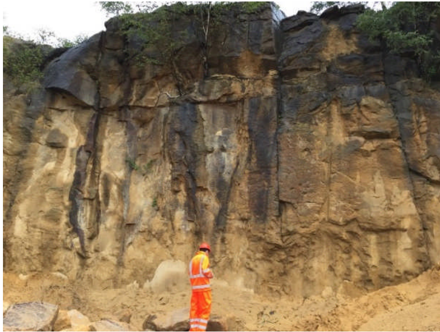
Figure 2.2 A set of near vertical incipient joints at Blackhill Quarry, West Yorkshire, UK. Note that rock materials are weathered predominately along joint traces, person for scale.
