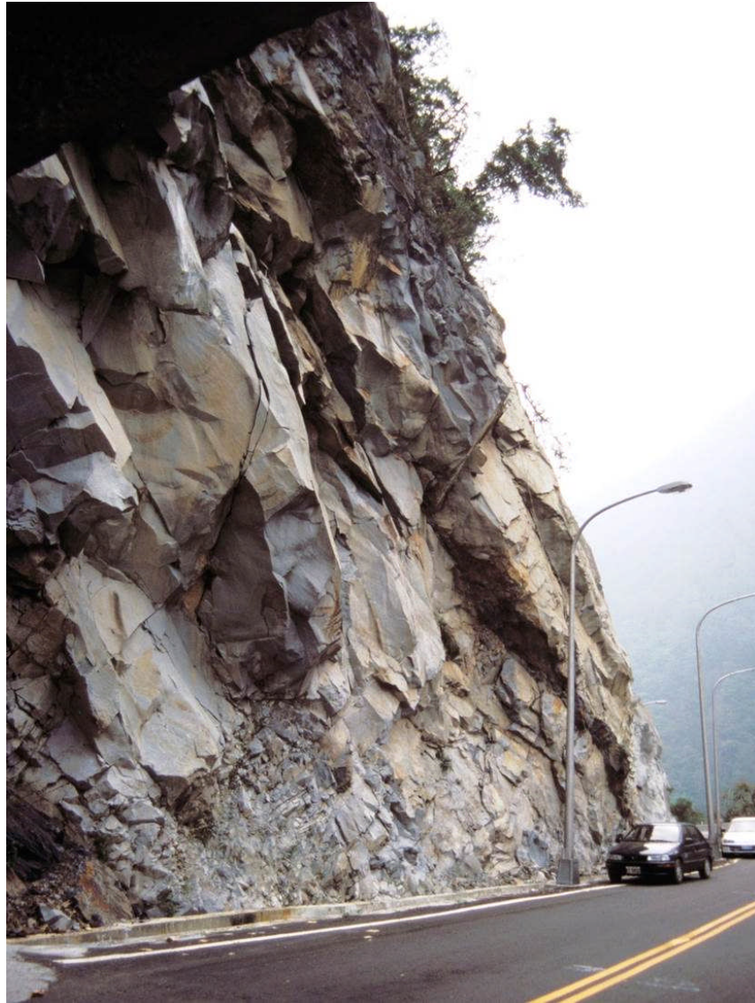
Figure 2.17 Slope with daylighting rock slabs threatening highway in central Taiwan. The incipient nature of the discontinuities contributes tensile and shear strength and allows temporary stability.
