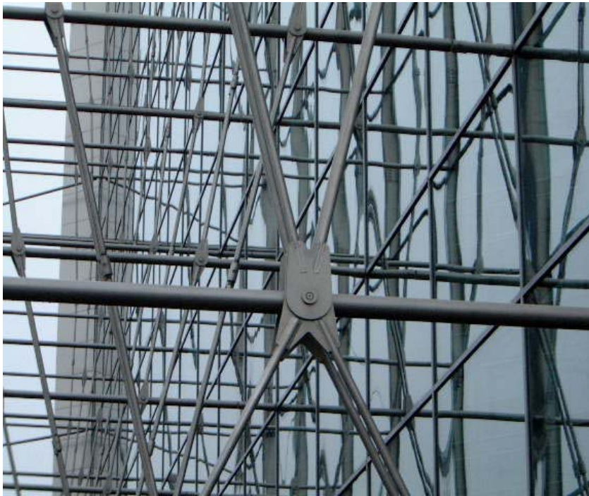
Figure 5 External stainless steel bracing system, Sanomatalo Building in Helsinki
