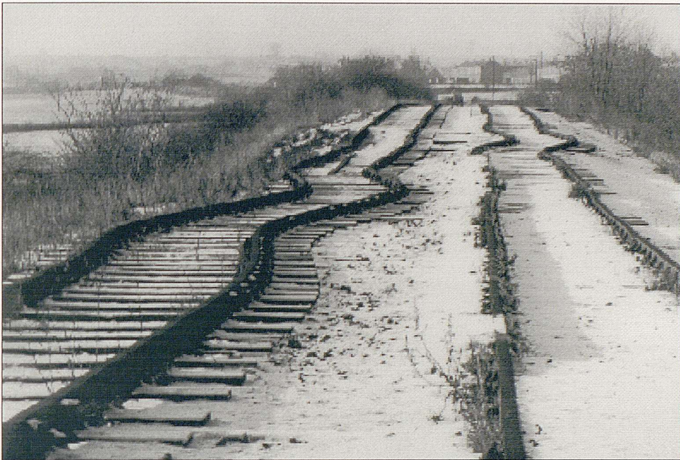
Figure 1.1 Localized buckling in a non-operational track caused by subsidence due to underground mining. (Source: British Rail, Derby)
