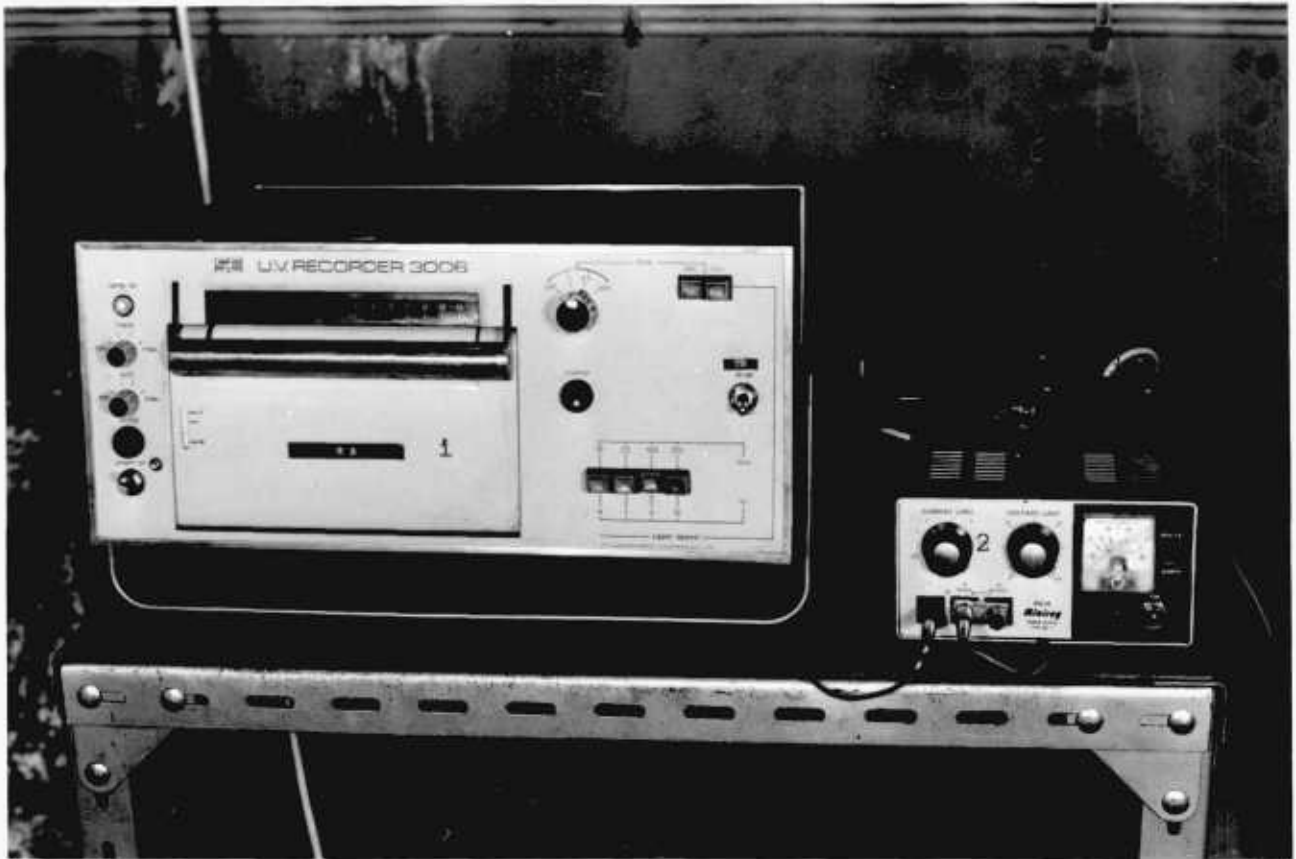
1.U.V.Recorder 2.Power pack 3.Junction box
