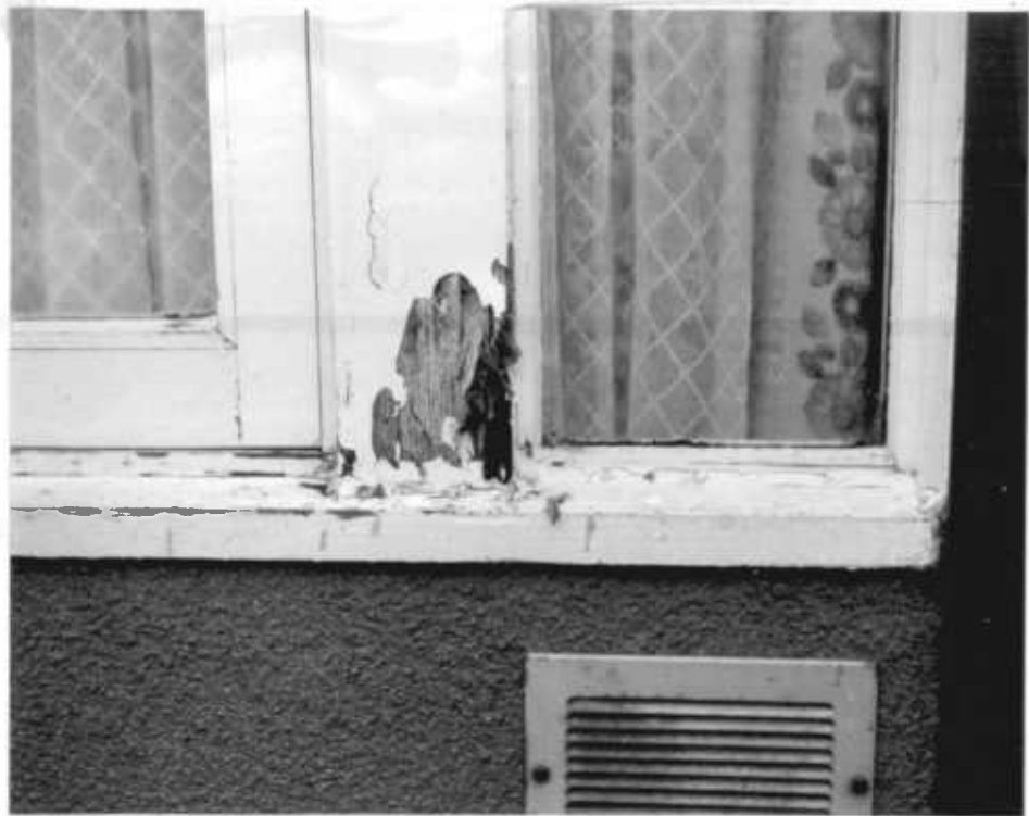
Fig 2.12 Larkhill; severe white rot at rail/stile joint
