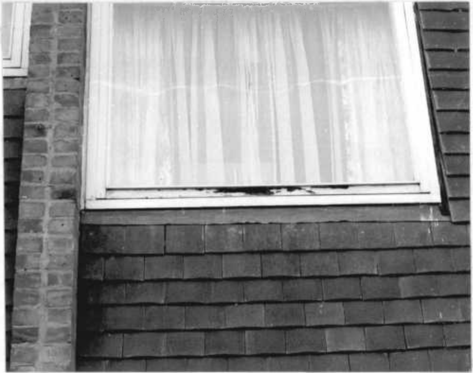
Fig 2.21 Chatham; decay in the centre of the bottom rail.
