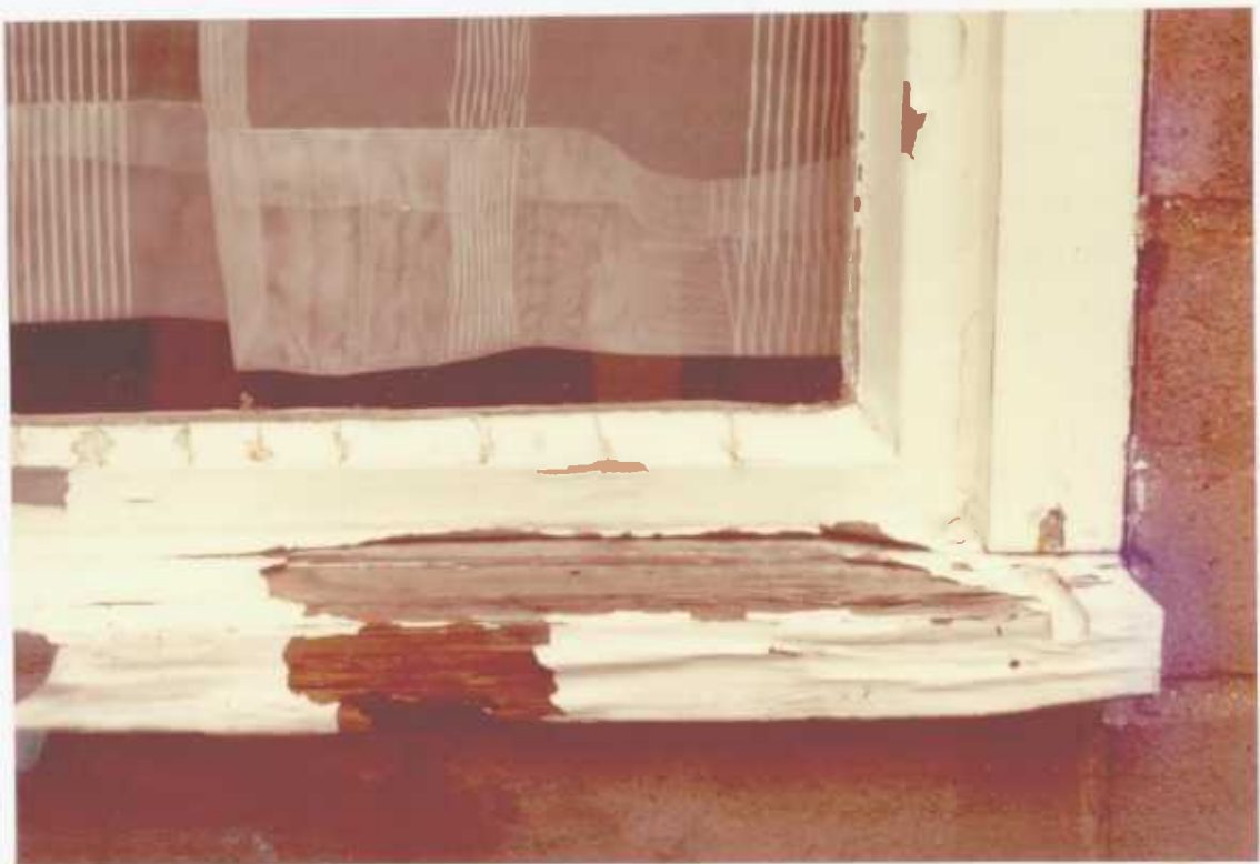
Fig 2.17 Cambridge; severe decay of sill associated with the water channel
