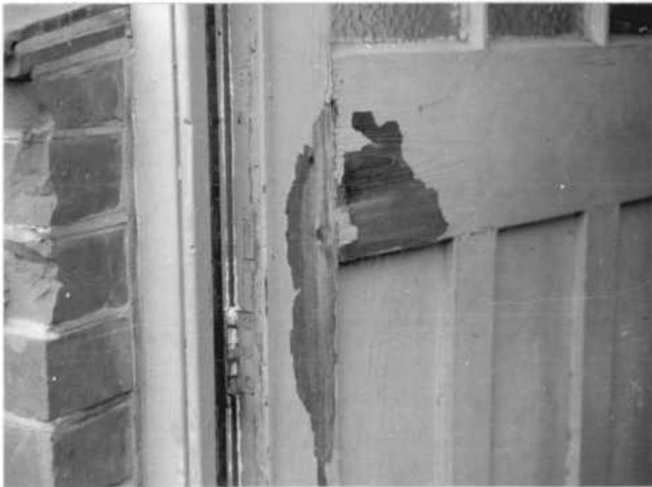
Fig 2.11 Larkhill; Noll Bingham road; a Scots pine door showing only slight decay after 45 years service.
