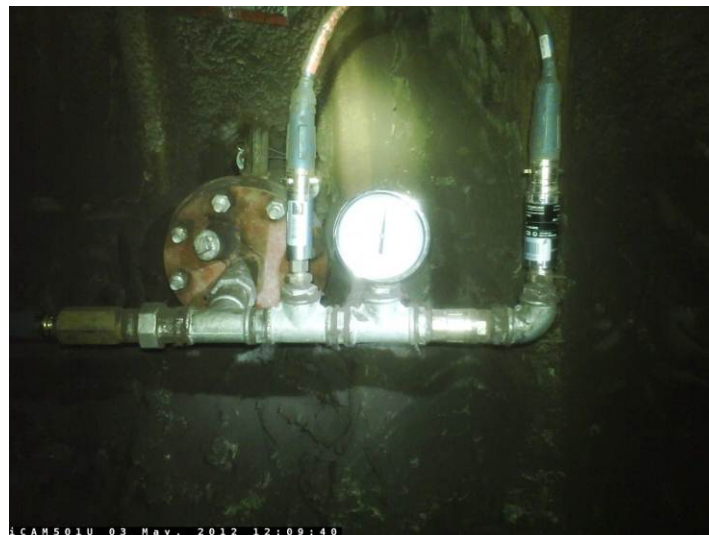
Figure A1.2: A completed pressure monitoring borehole on-site (Courtesy of Coal Mine Velenje researchers).
