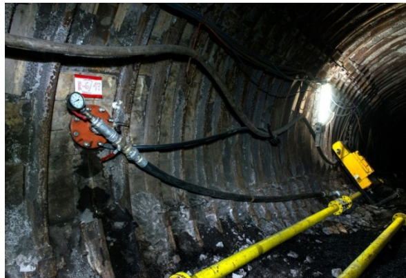
Figure 8.3: The connection between a drainage borehole and the pipeline at Coal Mine Velenje (Courtesy of Coal Mine Velenje Researchers).
