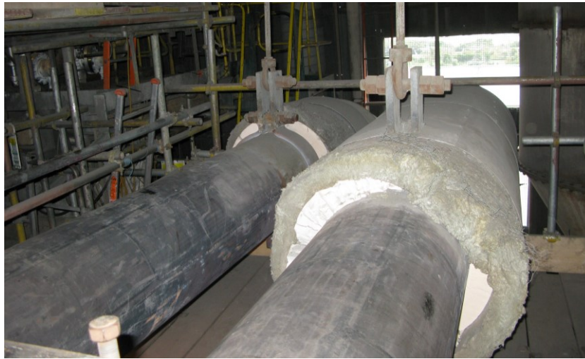
Figure 1.4: Photograph of CMV hot reheat pipes. Two pipes are shown during an outage. Hangers to suspend the pipes are shown in addition to thermal insulation which covers the pipes during normal operation.
