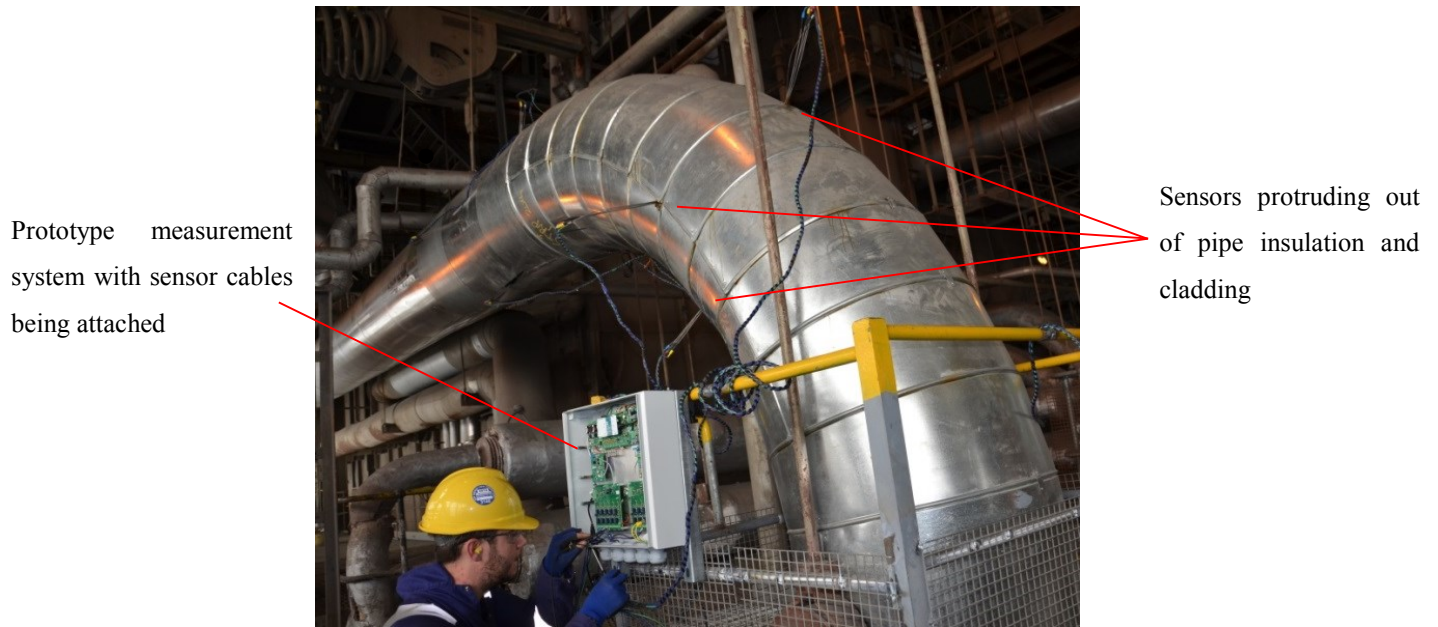
Figure 7.3: Photograph showing sensors and measurement system installed at West Burton power station.
