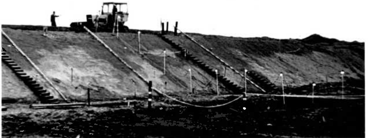
PLATE 5.8.1 INSTALLATIONS FOR TIME LAPSE PHOTOGRAPHY
