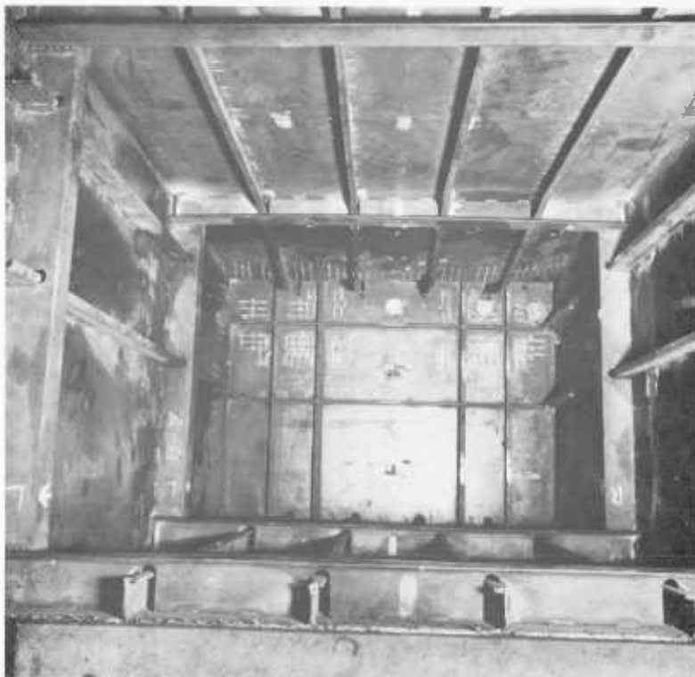
Fig. 2.14. Model 1 - an inside view of the model (from end A). Note the deflected shape of longitudinal stiffeners of the compression flange in the panel nearest to the central diaphragm and the lateral buckling in the next panel.
