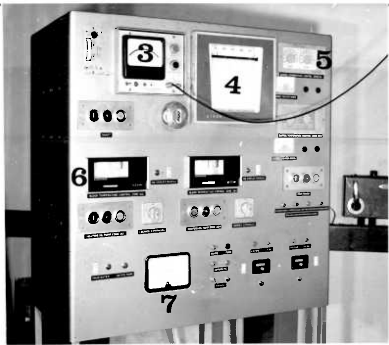
PLATE 2.6 - MAIN CONTROL CABINET
