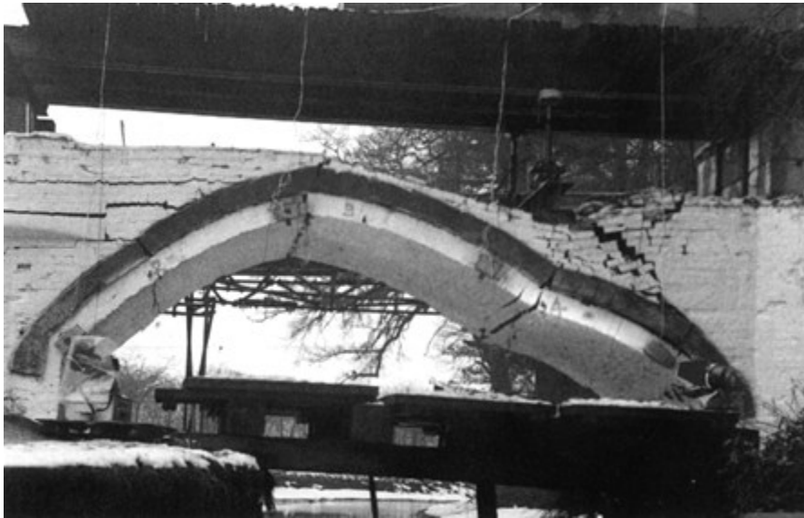
Figure 2-4: Collapse of the Prestwood Bridge due to a four-hinge mechanism (Page, 1993)
