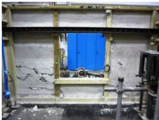
Figure 7. Damage state of the interior face at the end of test
