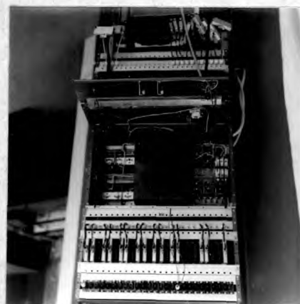
Fig.3.8 : Rear of Data Recording Unit
