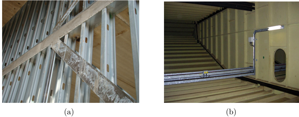
Figure 1.3: Thin-walled structures in civil engineering applications; (a) a typical thin-walled frame, available from http://www.sem.cee.vt.edu/research/thin_walled_structures.html , and (b) the Humber Bridge box-girder lower flange with stiffened plates.
