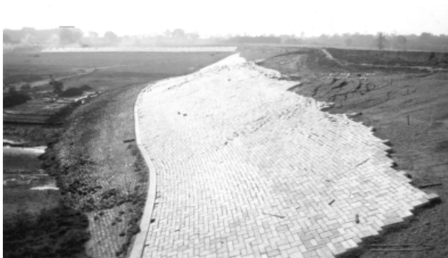
Fig. 4. General view of original dam failure. At the time of collapse the embankment was about 13.5 m high, and the slip involved a 175 m long central section of the dam
