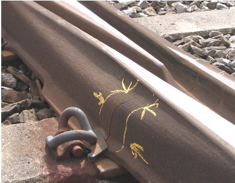
Figure 2-13: Cracked cast Manganese crossing.
