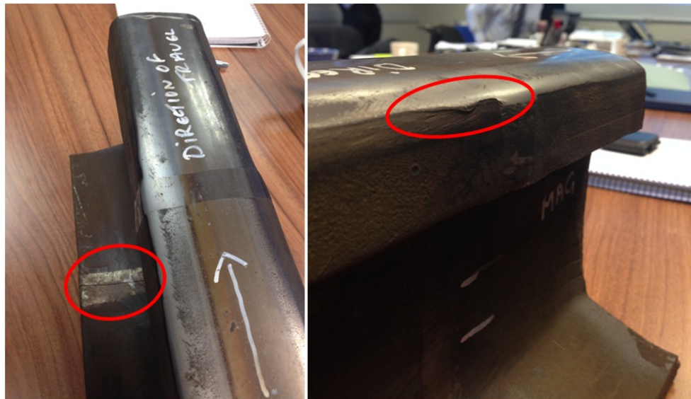
Figure 7-18: Cracked leg end weld and plastic deformation on a defective cast manganese crossing specimen
