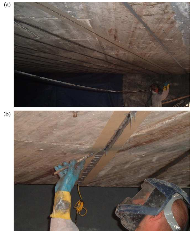
Fig. 2. (a) Grooves already cut underside of the bridge; (b) putting the rods into the grooves and gluing with epoxy.
