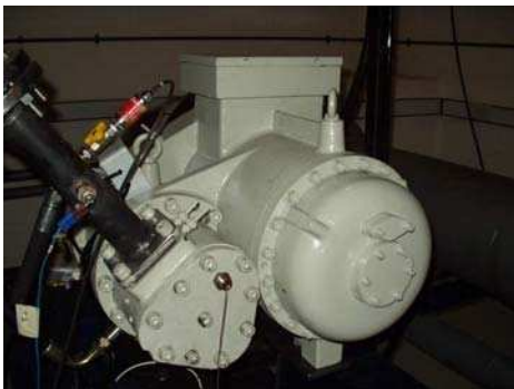
Fig. 6 Refrigeration compressor, Zhang et al, 2006
