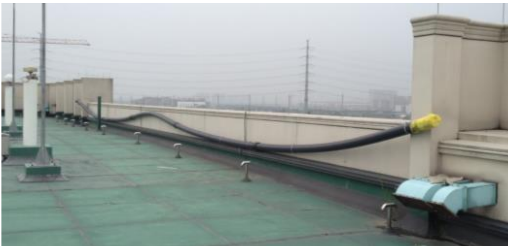
Figure 4 The test pipeline set up on the roof of the Science and Engineering Building at the University of Nottingham Ningbo, China.
