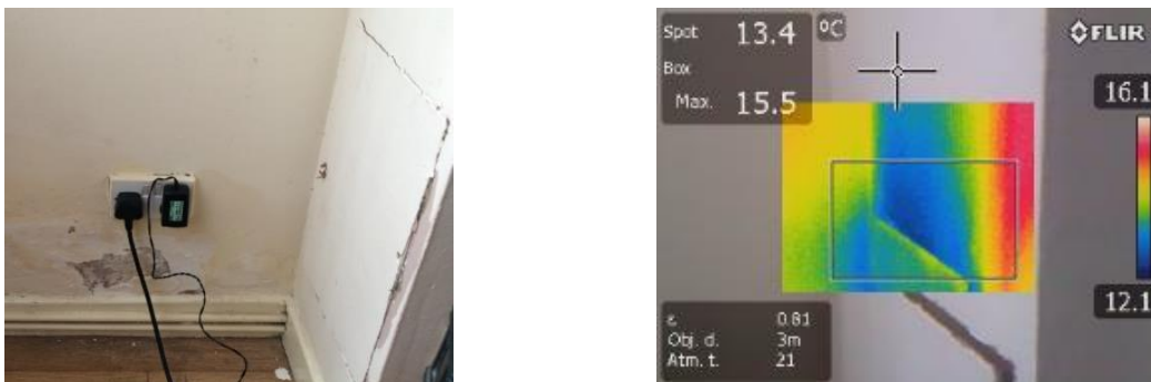
Figure 14: Photograph and thermographic image of a loosely installed plasterboard panel in house No. 2.
