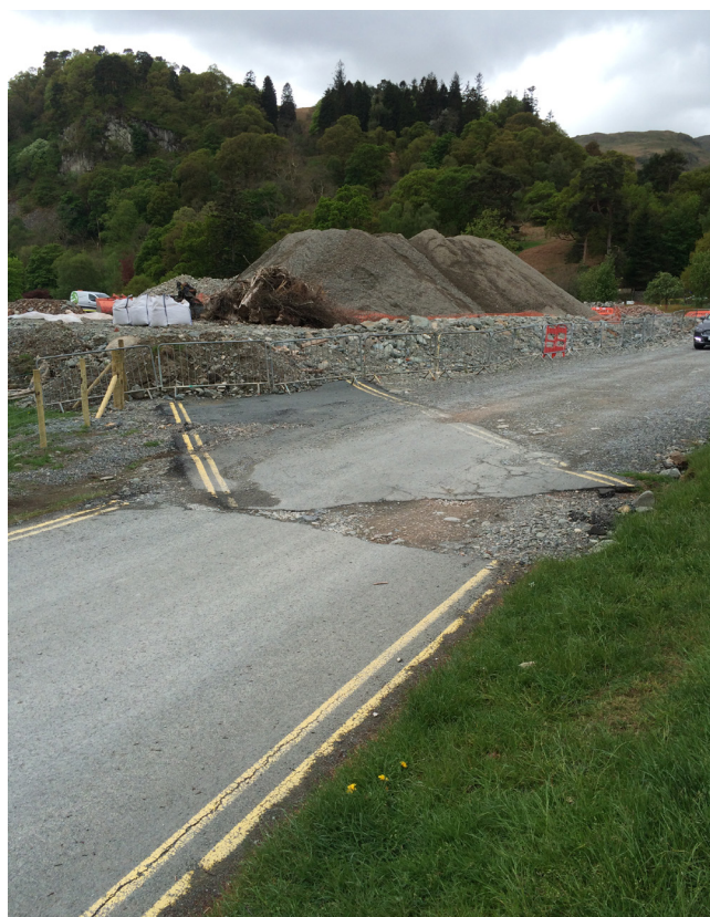
Plate 6 Road damage caused by flooding in Glenridding (Cumbria).
