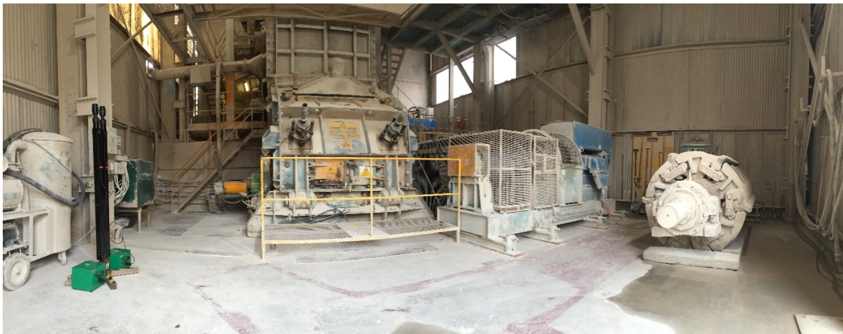
Figure 3 – Ballidon Quarry primary crusher shed with monitoring station shown on left hand side
