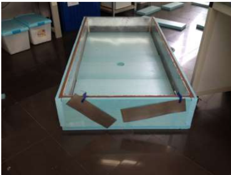
Figure 5-1: Test cell under construction-XPS boards are being attached to the stainless steel box
