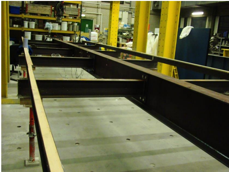
Figure 9 Outrigger beams used to support the decking to mimic un-propped construction (props used to stabilise the beam but were removed immediately after concreting)
