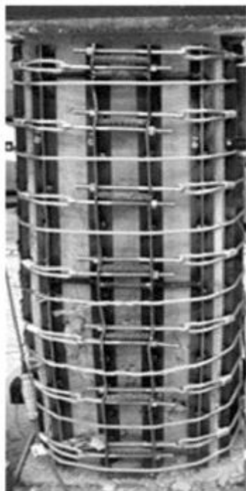
(c) Lateral buckling of T-shaped steel plates
