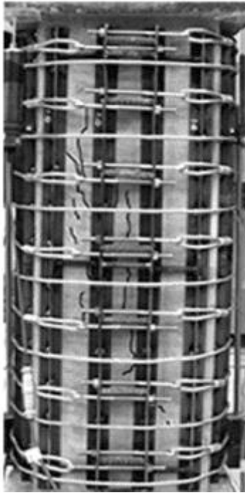
(a) Crack propagation at cover concrete
