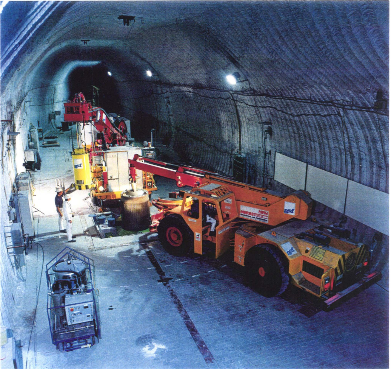
Fig. 29: Underground Disposal and Retrieval of the Canisters; Components Shown; Gallery Transport Vehicle, Borehole Slider, Single Transport Cask, Asse TB1, Disposal Machine with Shielding Bell; STC Still Handled with the Load Hooking Device
