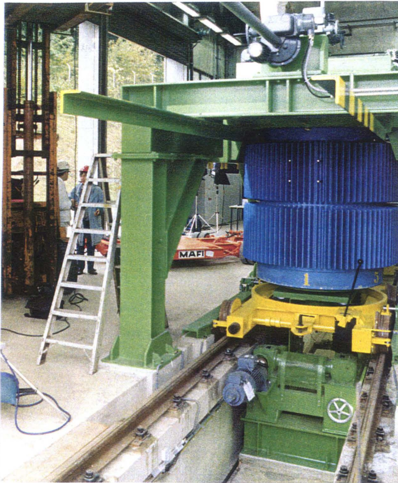
Fig. 20: Docking of the Multiple Transport Cask, Castor GSF-5, at the Transfer Station; Hoisting and Rotating Device Visible in the Pit between the Rails; MTC Raised from its Seat in the Carriage
