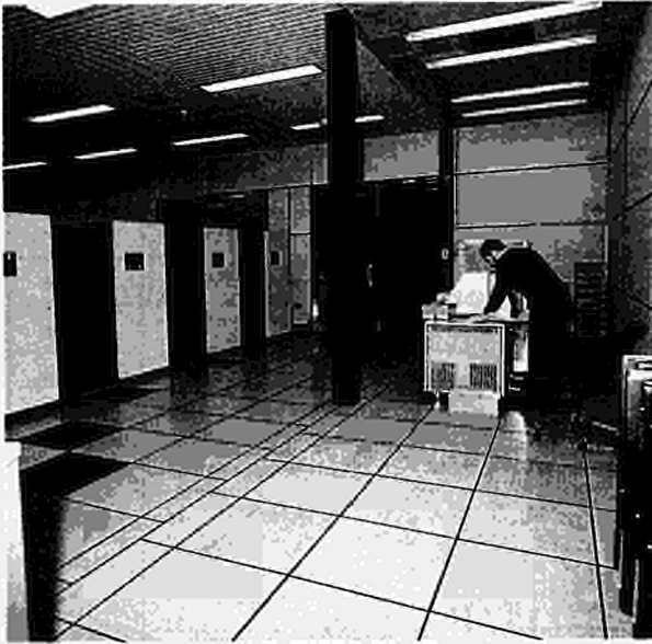
Fig.62: Installation of the IBM mainframe computer in the Building J2 computer room.
