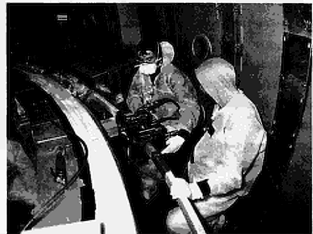
Fig.20: Coil No:D1 and Coil No:D4 copper bar conductor being brazed inside the JET vacuum vessel
