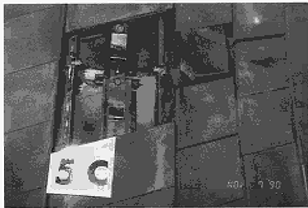
Fig.11 Damage at the inner wall
