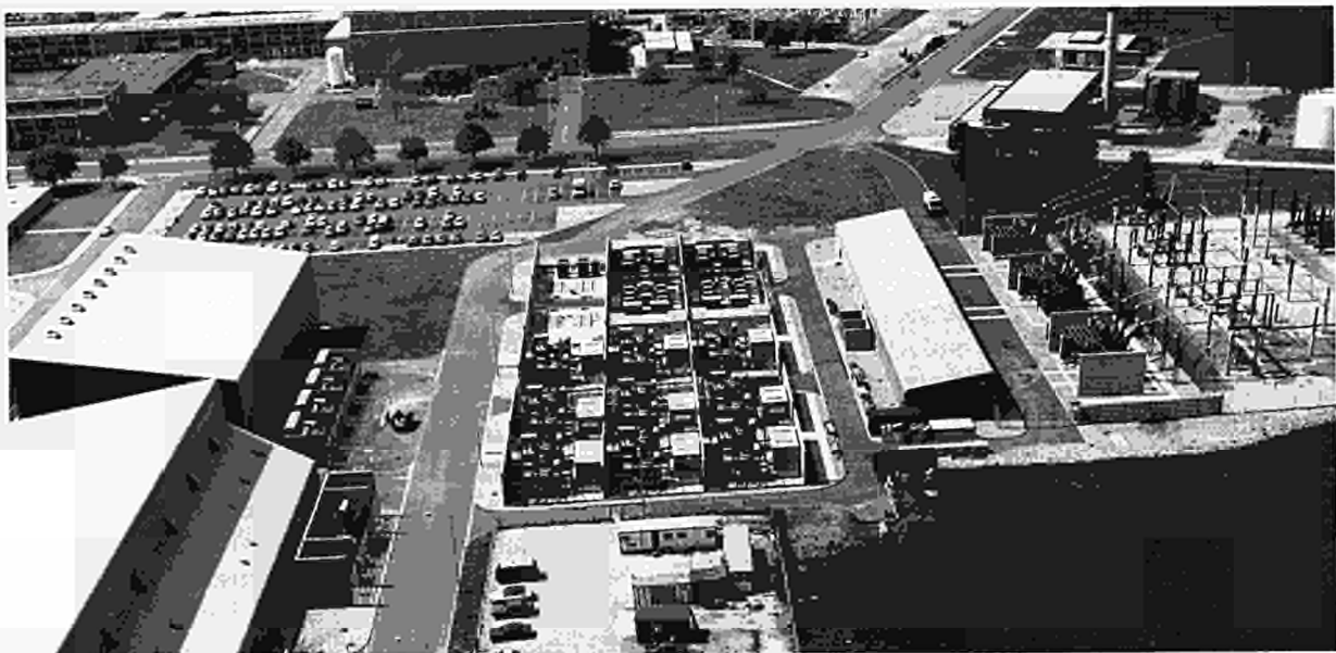
Fig.20 Outdoor AC-DC high voltage power supplies for neutral beams and ICRH. The bays for the LHCD power supplies are also shown.
