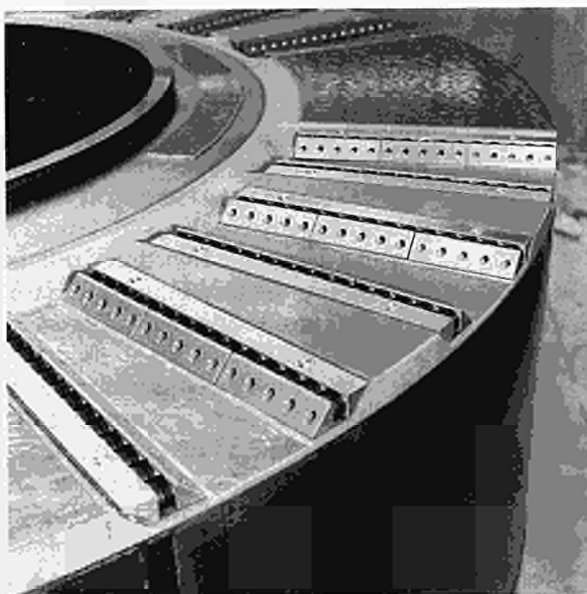
Fig.17 Assembly of the new spring keys between the P1 subcoils to improve electromechanical behaviour during operation.
