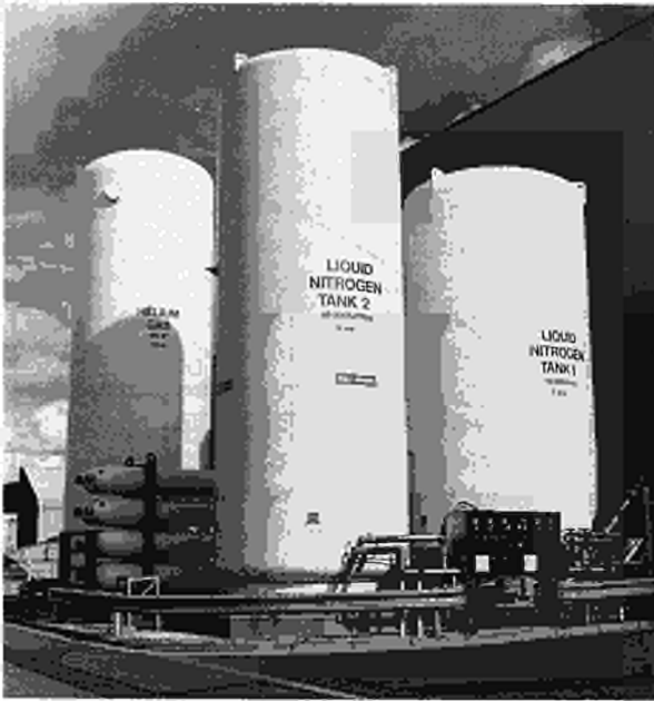
Fig.23 Upgraded Cryosystem showing LN 2 tank, LHe buffer tank, and high pressure storage cylinder;
