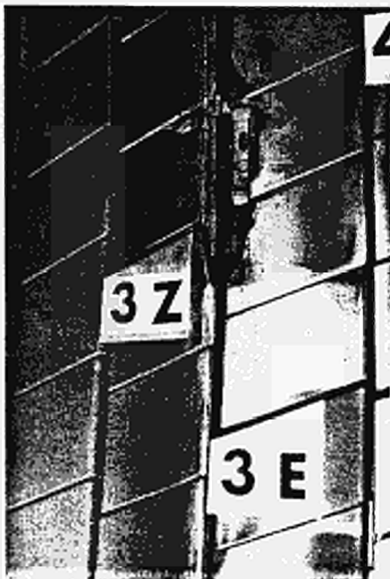
Fig. 5: Damage to the tiles at mid-plane of octant-joint 3/4. This is the most severe damage which occurred and is due to impinging high energy runaway electrons generated during disruptions.
