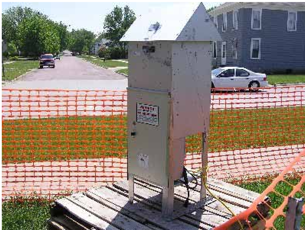
Photo 1 – West Site Perimeter Air Monitoring Station
