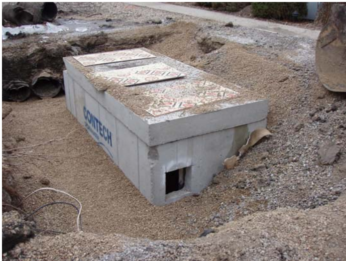
Grit Collection Chamber (Site H8)
