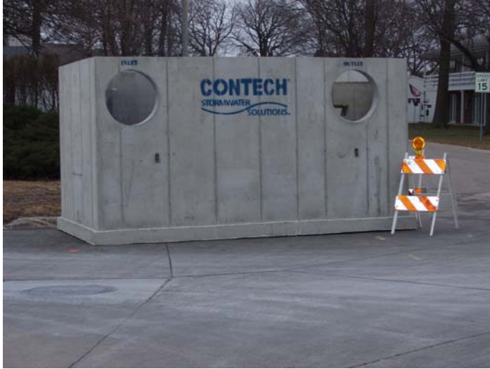
Grit Collection Chamber (Site G4)
