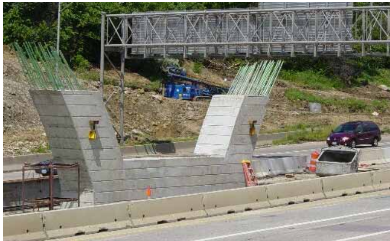
Figure 3.15. Center pier after formwork was stripped and before reinforcing steel and formwork for the pier cap were constructed
