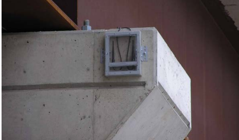
Figure 4.18. Data acquisition sub-system WAP antennas placed at the edge of bridge pier
