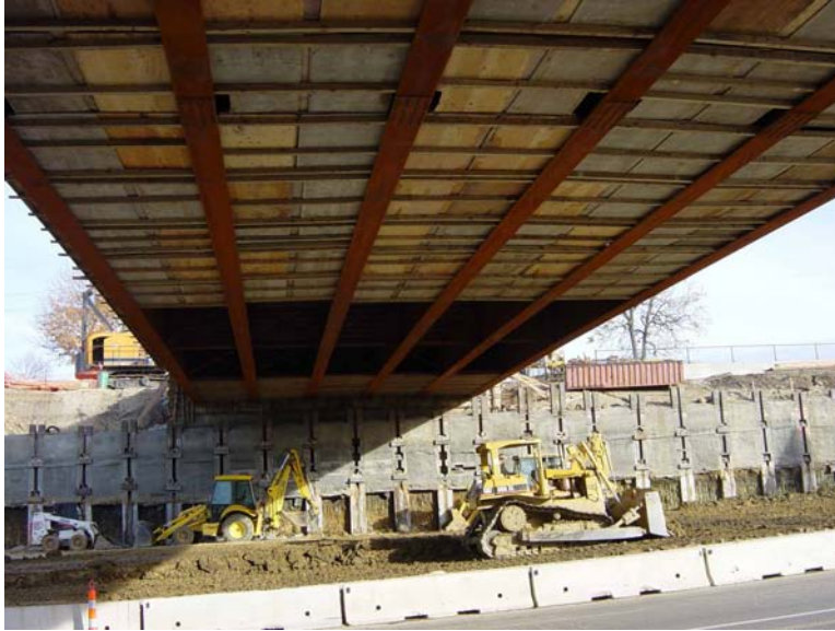
Figure 3.23. Work platform resting on the bottom flange of the girders over I-235
