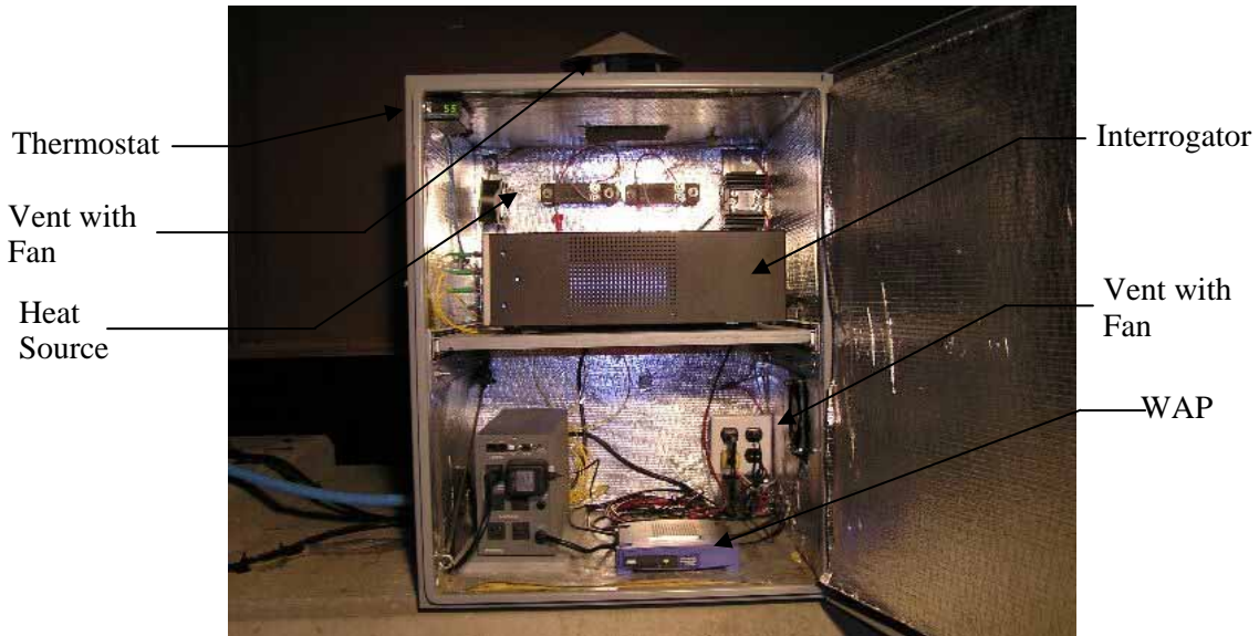
b. DASS equipment in steel cabinet
