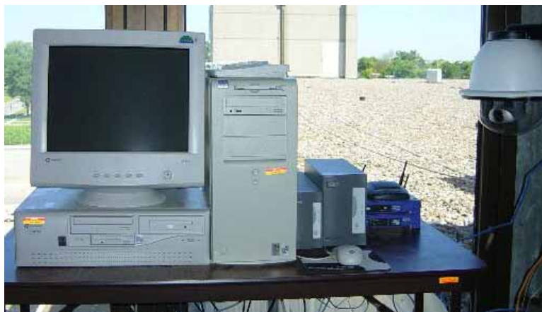
Figure 4.19. Gateway sub-system located in secure facility near bridge
