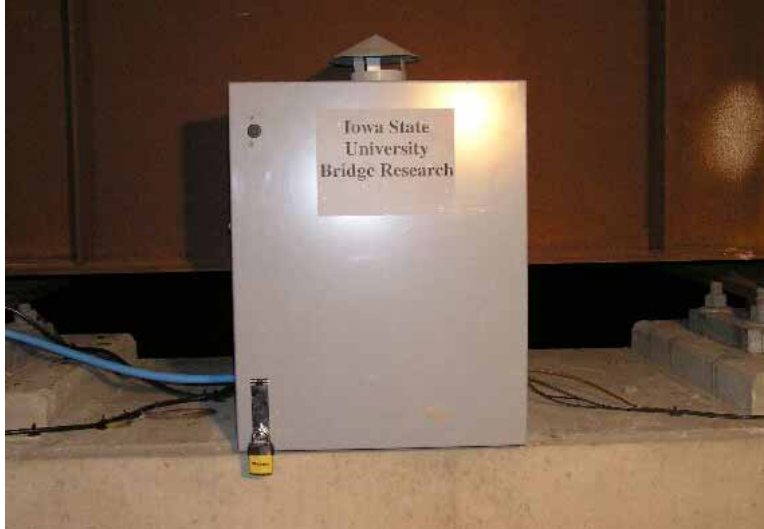
a. Steel cabinet
