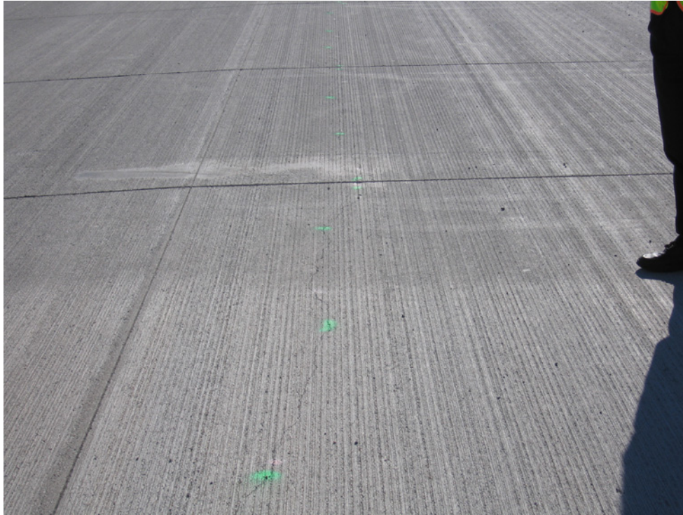
Figure 15. Random Longitudinal Crack in North Dakota Pavement
