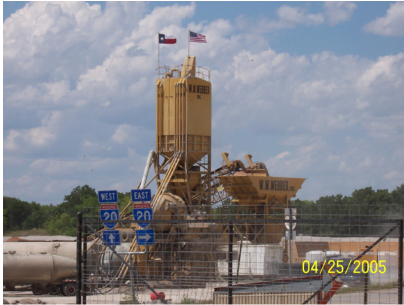
Figure C.14. Batch Plant near the Texas Shadow Project Site
