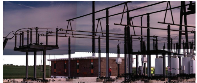
Figure 2-8. A substation survey that was performed using laser scanning technology. The total station captured images and placed the survey points on top of the image.
