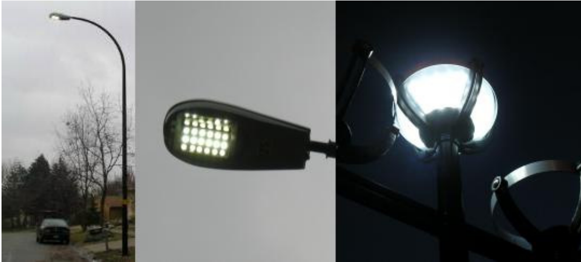
Figure 5-6: Cobra head (left and center) and globe LED lights evaluated in Ann Arbor (Image source: City of Ann Arbor, 2007)
