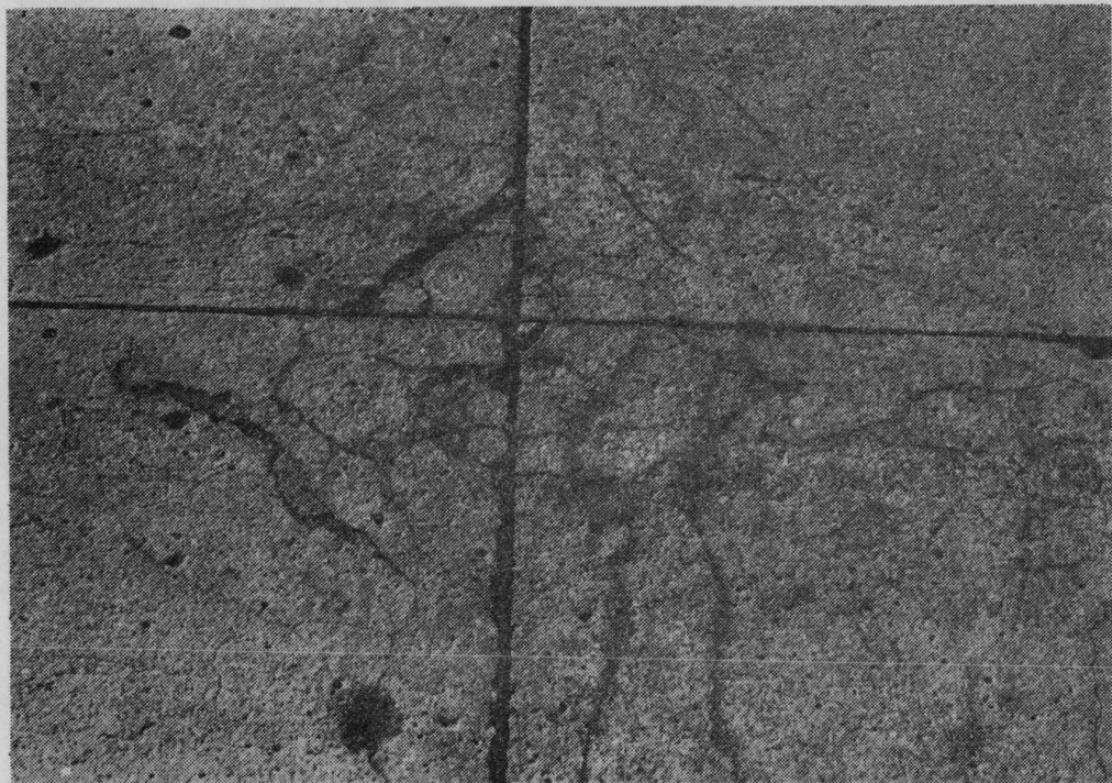
Figure 1 A close-up of D-cracking at the intersection of the transverse and longitudinal joints
