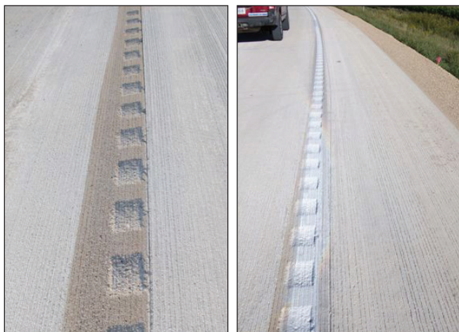
After milling (left) and with paint applied (right) (photos courtesy of Linn County)
